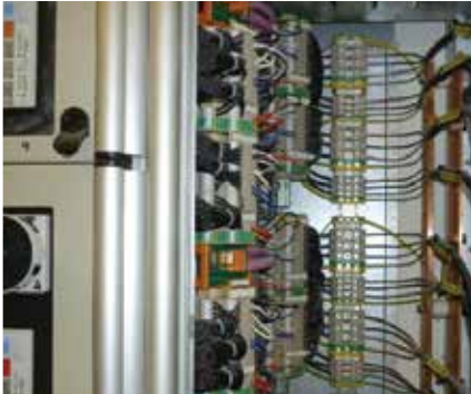
FEEDERS CABLE ROUTING – GULF CEMENT QATAR
