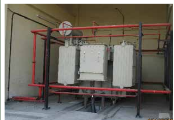
Aditya Birla WHRS – Distribution Transformer
