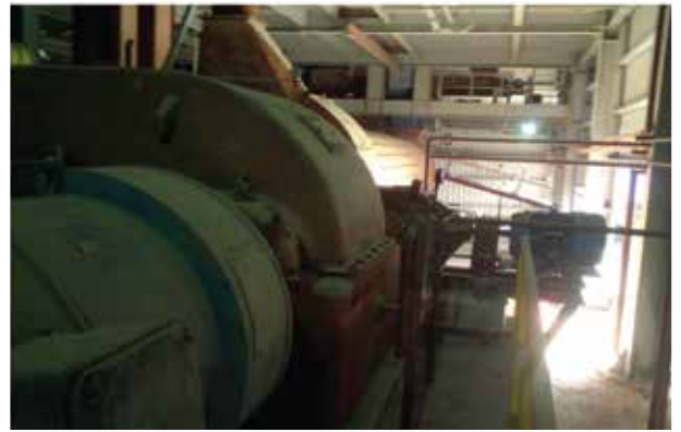
Abu Dhabi National Cement Factory Mill & Separator Drive
