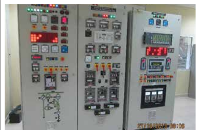
Aditya Birla – WHRS -Turnine control and Automatic Synchronisation Panel
