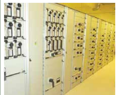
SUBSTATION – GULF CEMENT QATAR
