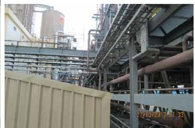
Aditya Birla WHRS – Cable Cellar & Cable Trays
