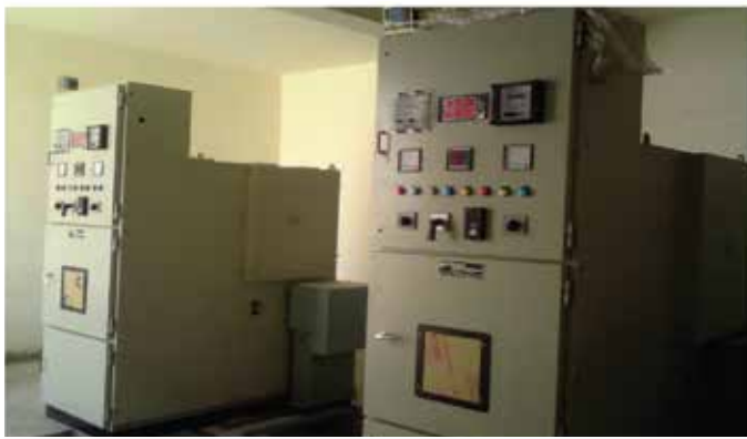
Abu Dhabi National Cement Factory - Substation
