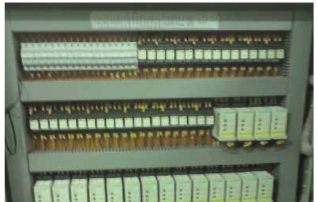
Abu Dhabi National Cement - Softstarter & Distribution Panels
