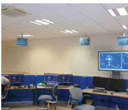
GULF CEMENT QATAR – CCR – X RAY LAB & ROBO LAB
