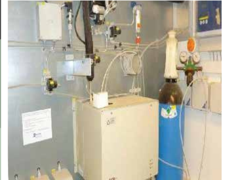
KILN INLET ANALYZER ROOM AND PROBE – GULF CEMENT QATAR
