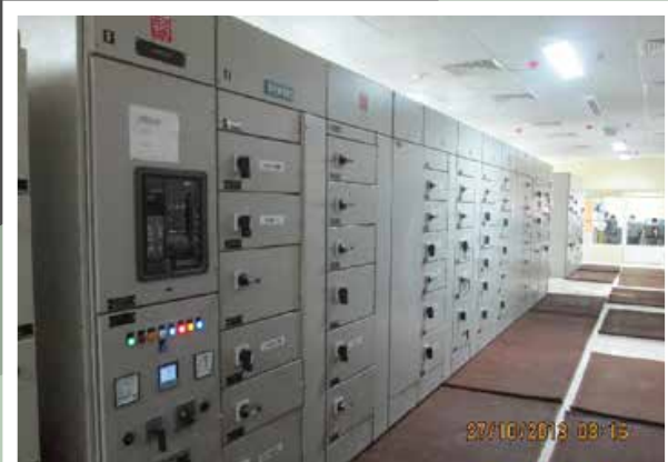
Aditya Birla WHRS – SUBSTATION
